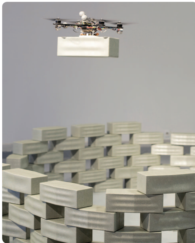
FIGURE 10 Placing a module. The vehicle hovers above the structure before placing a construction module. A vertical trajectory that results in the foam element impacting the structure at 1 m/s is executed to place the module. The actual mean impact velocity was 1.04 m/s with a standard deviation of 0.02 m/s. (Photograph by Franois Lauginie.)
